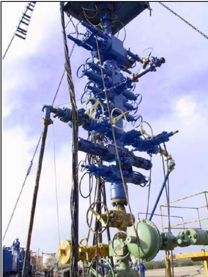
Figure 8-1. Pressure Control Equipment for a CT Operation
