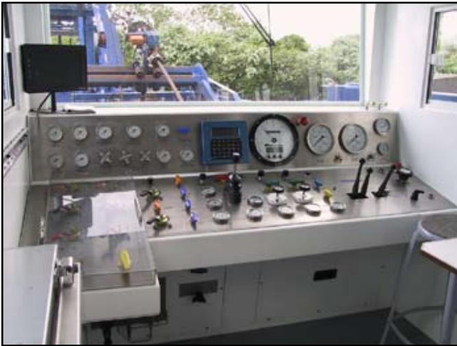
Figure 5-2. Controls and Gauges to Operate CTU Components
