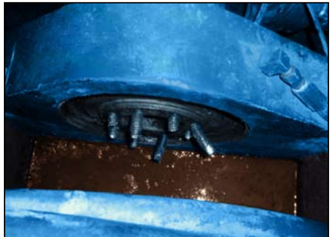
Figure 6-22. Damage Caused by Incorrect Torque on Swivel
